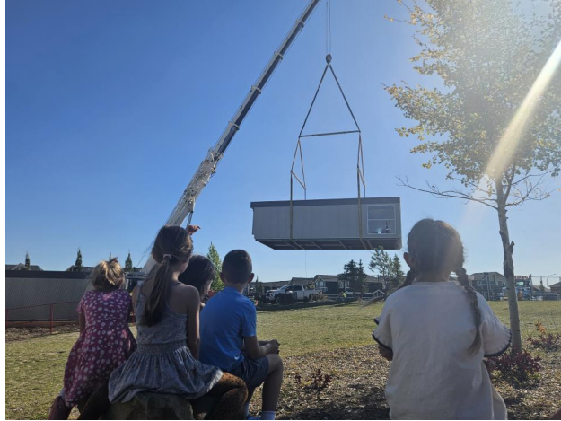
1 - A few of our Grade One students in Mr. Cox's class witnessing the portable install.
